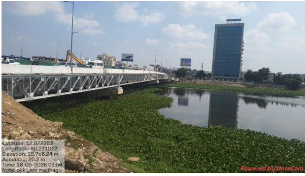
Fig 3 — Okkiyam Maduvu bridge blockage, 18-05-2026. GPS: 12.922953, 80.231012
