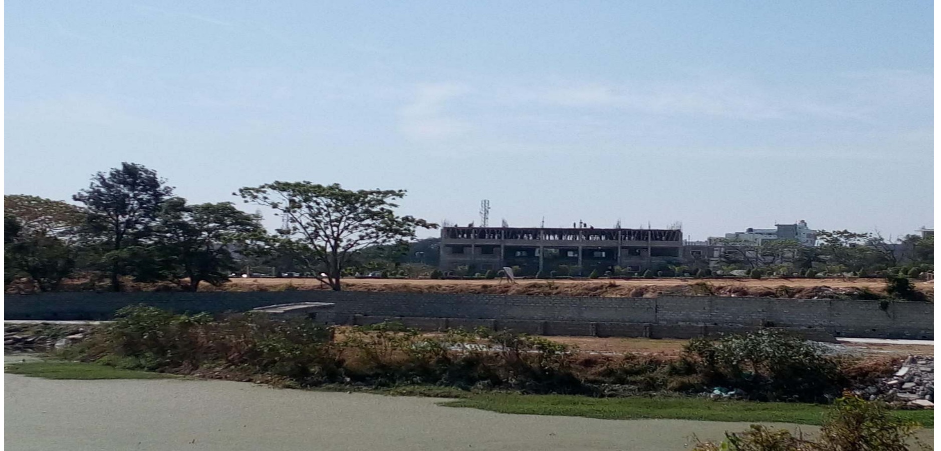
A compound wall has now come up around this encroached water body complete with a shed for a worker to stay. (February 2018)
